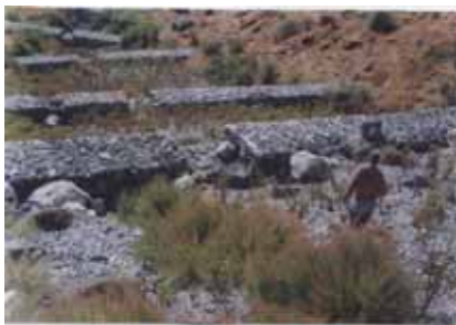
Well stabilized check dams
