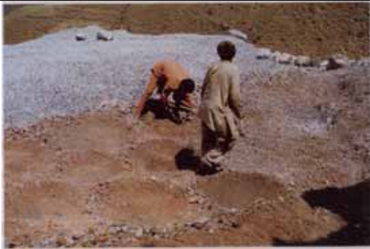
Rehabilitation work in progress at Top Bench of M/s K.K. Anand's Mine
